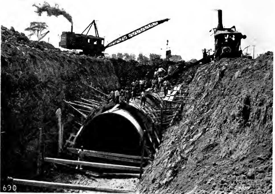
A BUCYRUS DRAG-LINE BACKFILLING ON THE WETHERBY SEWER, DETROIT, MICH. Blaw-Knox collapsible steel forms are being used on this job by the contractors, Nash Brothers, Chicago, Ill.
